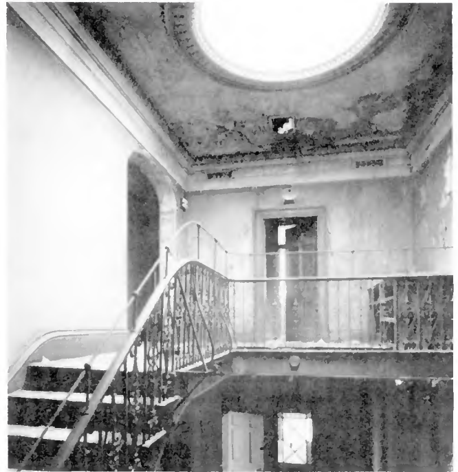
Top landing of The Priory, c 1825, demolished 1968. Reproduced with permission of the GRO (ref D3867/IV/35 DNC5-26).
