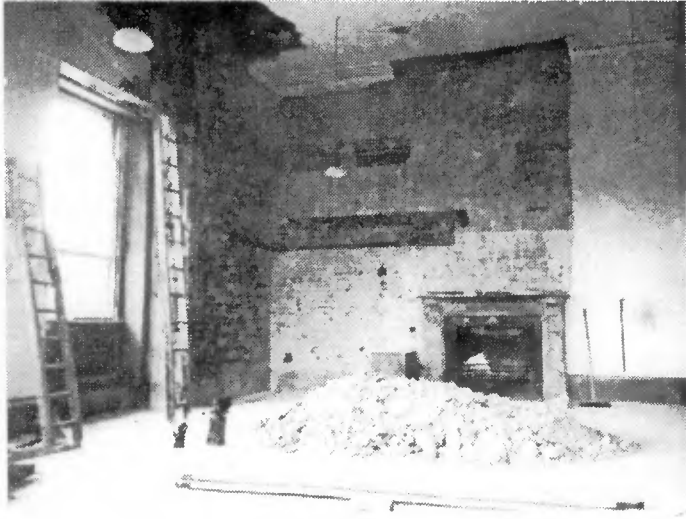
Removal of plaster to expose the dry rot
